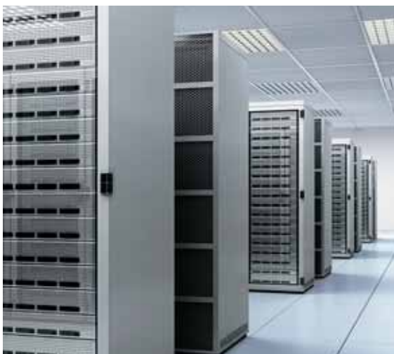
POWER MANAGEMENT & MULTIMARKET
